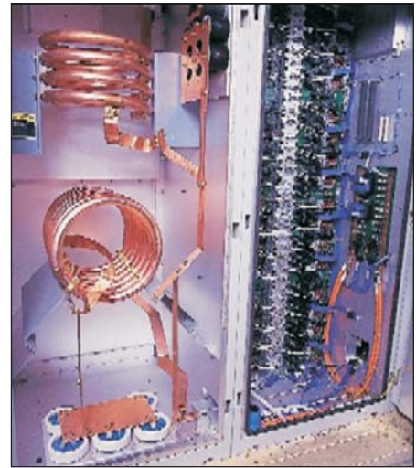
Figure 16 · Output section of a 50-kW AM broadcast transmitter. (Courtesy Harris)
